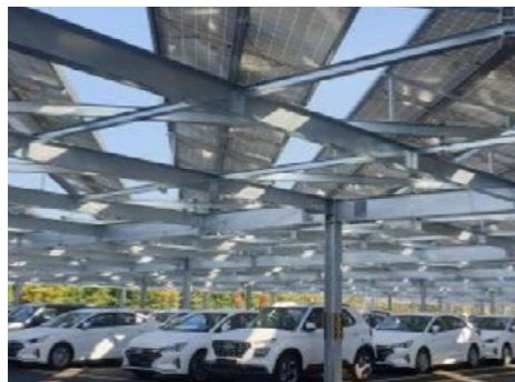
A photovoltaic power generation facility in the parking lot of the Ulsan Plant's driving test site
